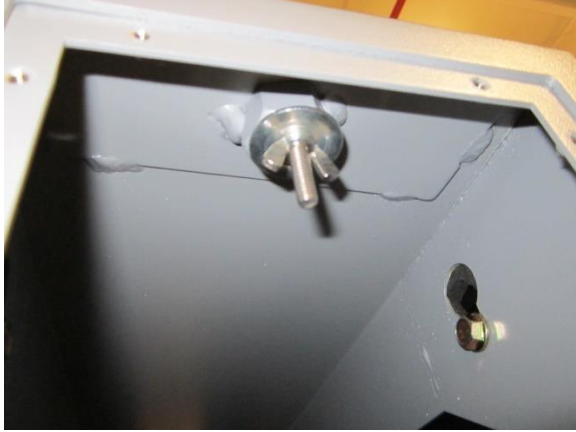
Hole Sealed by the Hole Cover
