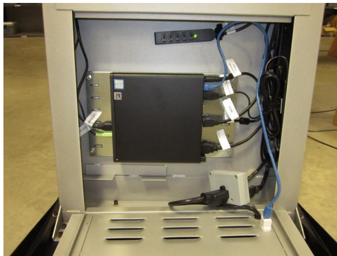
Computer Mounted in Louver Area
