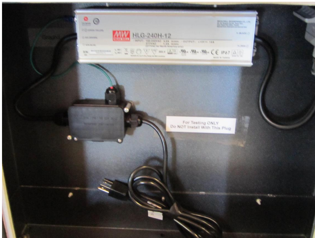
Test Cable in Kiosk. WARNING: DO NOT USE AFTER INSTALLATION
