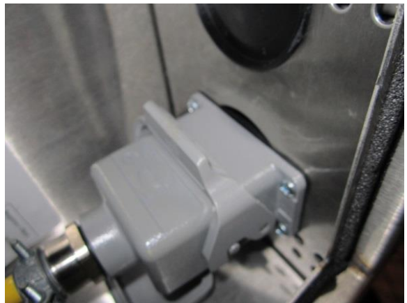
Power Connected and Locked
