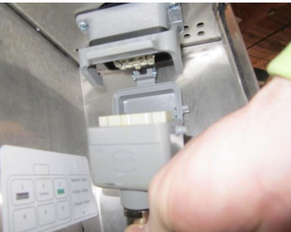
Disconnected Large Power Connector
